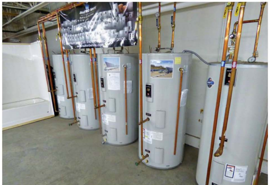
Bradford White water heaters are installed at Michel Sales training center that the company expects will host nearly 800 trainees in 2016.
