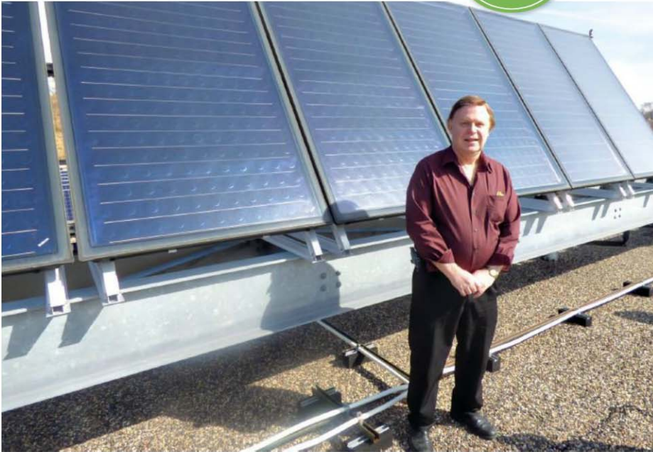
Harold Bruner, P.E., is one of two in-house engineering experts for Michel Sales Agency. He designed the solar hot water and radiant systems at the company's headquarters.
